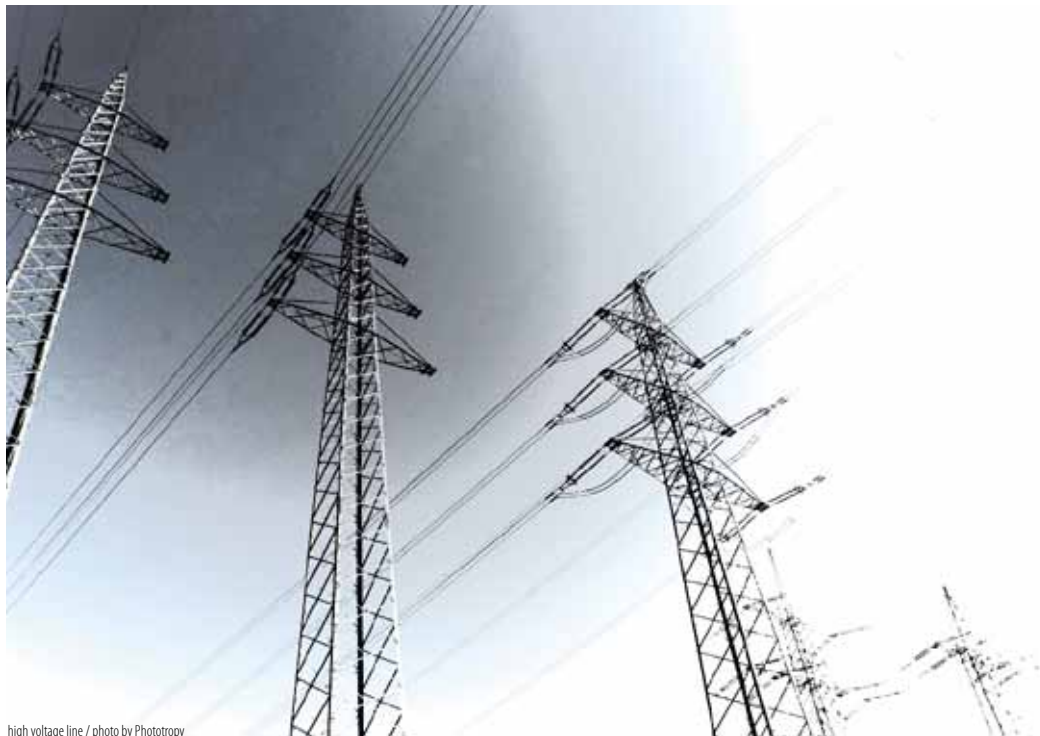
high voltage line / photo by Phototropy
